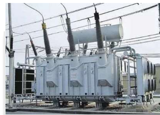
Ultra High Voltage Transformer
